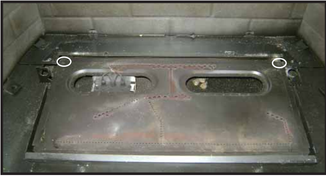
Figure 3.8 Remove Screws from Burner Assembly Rear Corners
