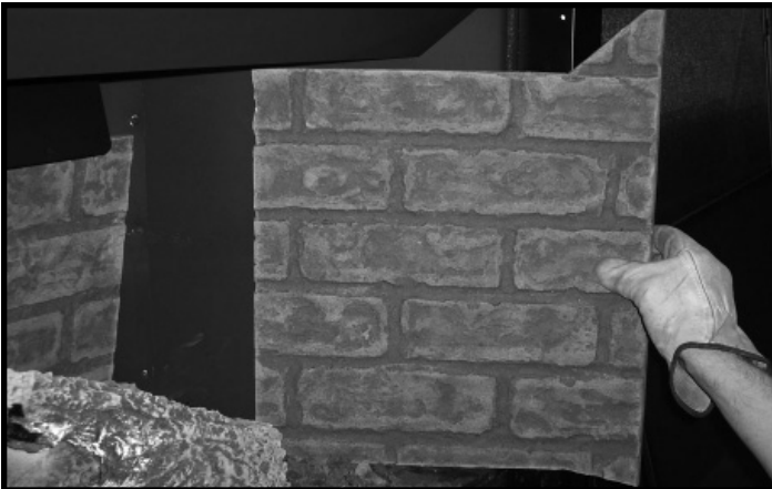
Figure 8 Position Side Refractory
